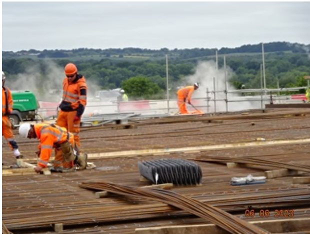
Photo of Silica dust being kicked up by workers on site
