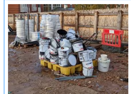
Potentially hazardous substances piled up on live site.
