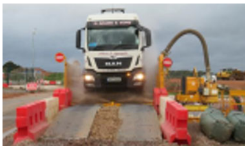
Wheel Wash Unit (WWU) for Vehicles leaving site.
