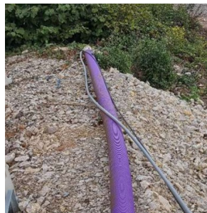
Exposed cable left near vegetation.
