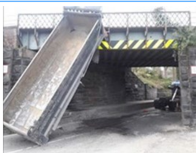
Photo of wagon colliding with bridge deck and become dislodged – view from road.
