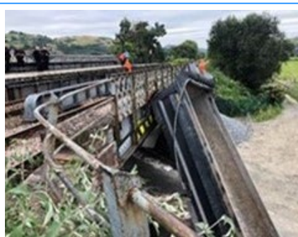
Photo of wagon having collided with bridge deck.
