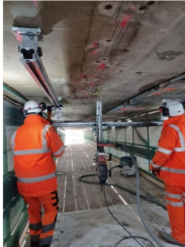
Figure A2 A drilling rig can be used to eliminate the MSK demands of drilling holes overhead (Photograph courtesy of Concrete Repairs Ltd (CRL))
