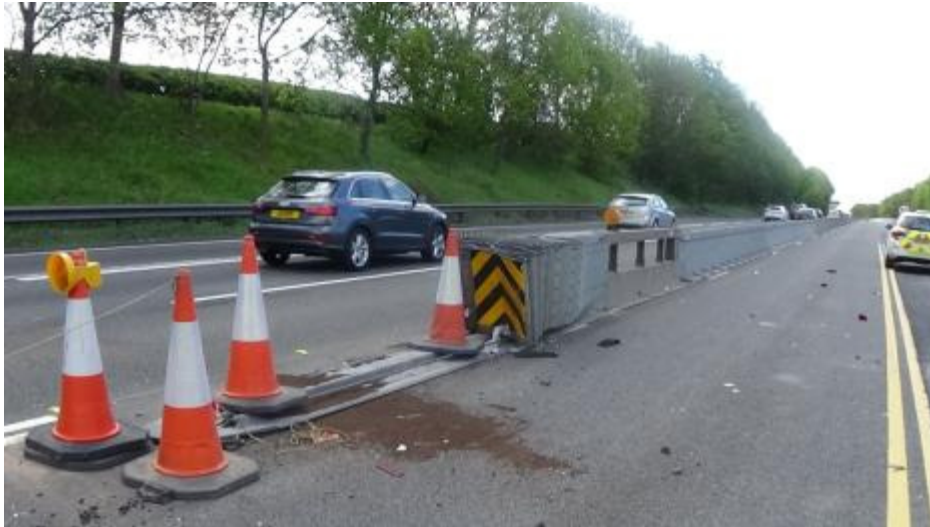
Photo.2 Damaged Crash Cushion terminal
