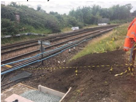
Safe access for temporary works?
