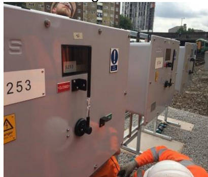
83kg but needs a four-man lift to move it!
