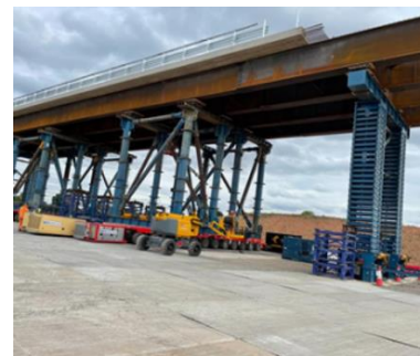
Offline bridge construction, built at ground level, jacked and moved into final position using SPMTs (self-propelled modular transporter)
