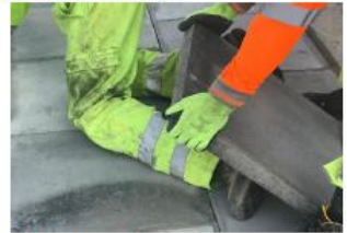
Suspected slab position on operative
