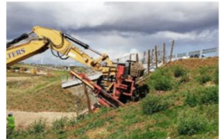
Overturned plant on side slope
