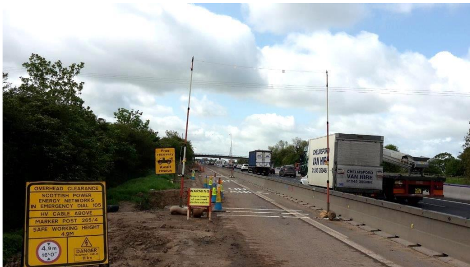
New signs have been made and placed on site, they state whether it is cables or structure above, outlines the minimum safe clearance height, identifies the marker post location, and emergency contact 'DIAL 105'.
