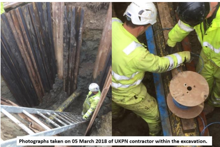
Photograph of the collapse taken on 07 March 2018.
