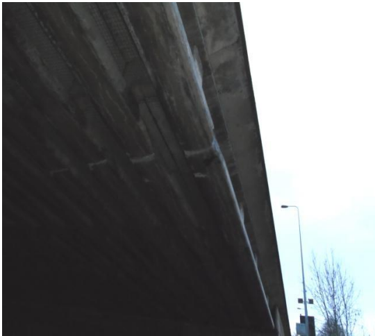
(Underside of bridge deck showing damage)
