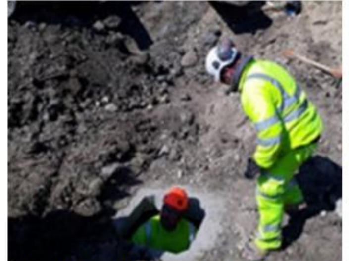
Photo of site worker in confined space without the correct precautions.
